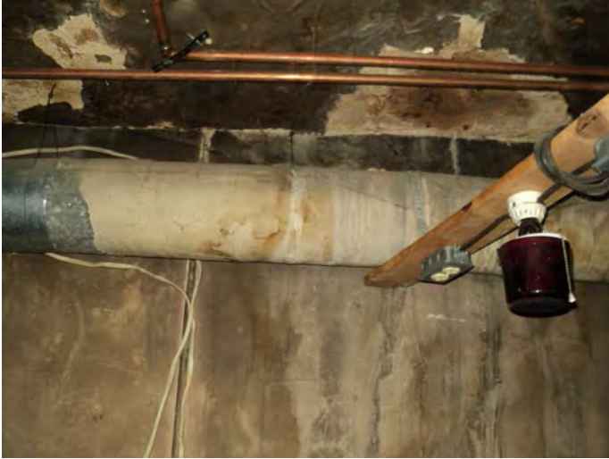
1. Insulation wrap around duct work in workshop/garage.
