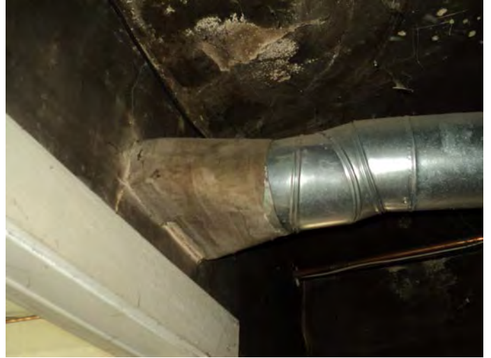
2. Insulation wrap around duct work in workshop/garage.
