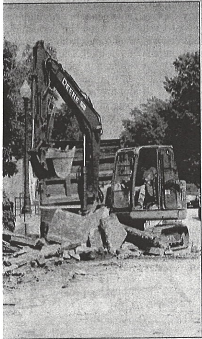
A section of sidewalk on Main Street in Warren is being demolished as an excavator rips out layers of concrete last week.
