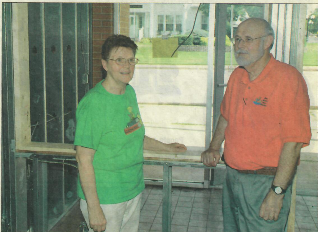
St. Clair Scenic Regional Library Librarian Karen Fogelbach, left, and Scenic Library System Director Ken Rohrbach look over the construction work being done on the local library's soon-to-be new location at 515 E. Springfield Road. Missourian Photo.
