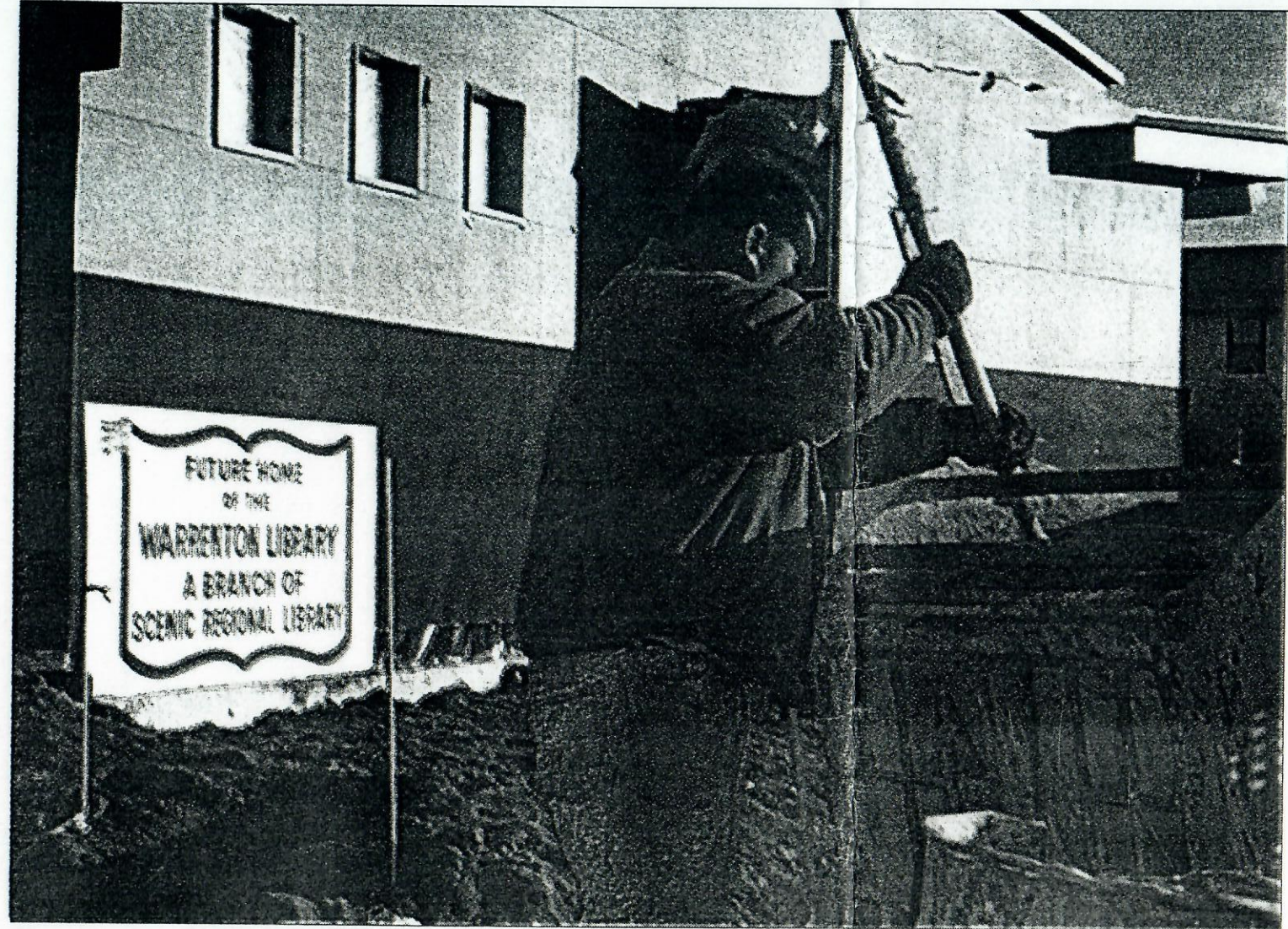
Matt Richardson, a worker for Mike Zekoll Masonry in Jonesburg, mixes mortar Feb. 6 for the brick exterior walls of the Scenic Regional Library in Warrenton.
